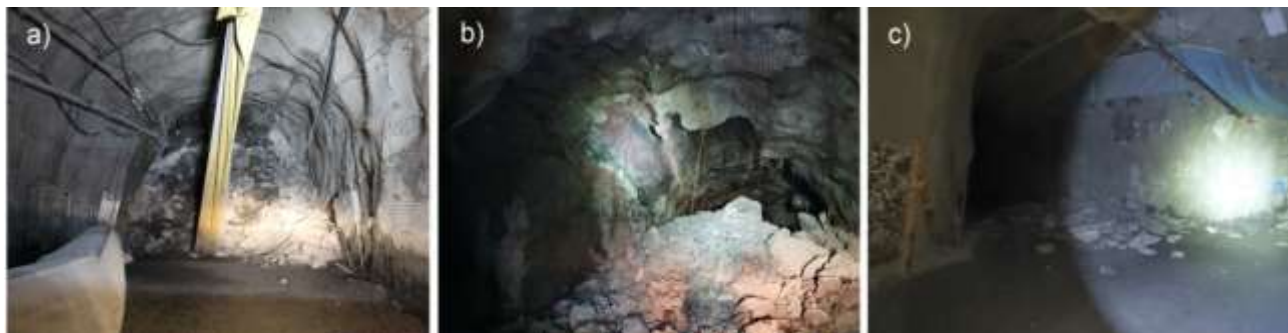
Figure 5. Examples of severity of damage: (a) Heavily damaged area; (b) Area of major damage; (c) Area with the localized damage, Boskovic (2022).
