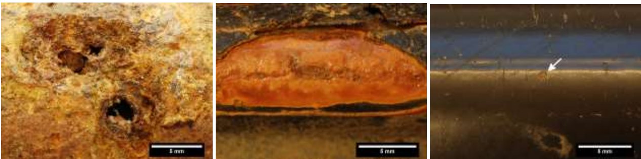
Figure 20. Observed corrosion types along the bolt length: a) general corrosion, b) pitting corrosion and c) pinpoint rusting, Hadjigeorgiou et al (2019).
