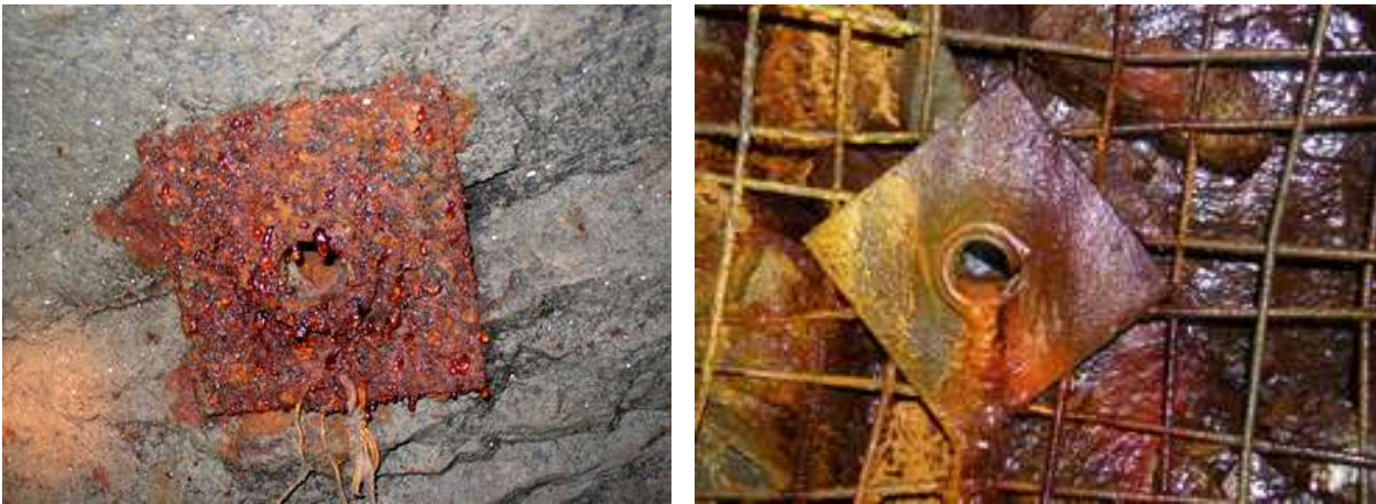
Figure 19. Friction rock stabilizers showing signs of a) atmospheric corrosion; b) aqueous corrosion.
