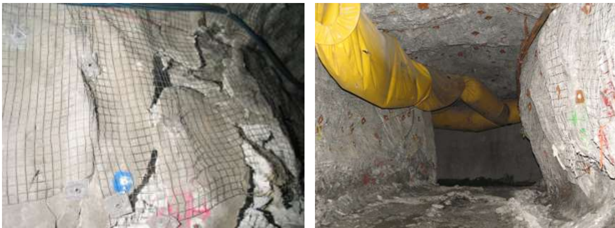
Figure 16. a) mesh overlaying fibre reinforced shotcrete; b) welded mesh, Potvin and Hadjigeorgiou (2008).
