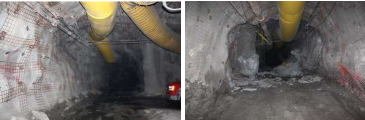
Figure 7. a) Rehabilitation following the 2009 event; b) Damage following the 2011 event, Counter (2014).
