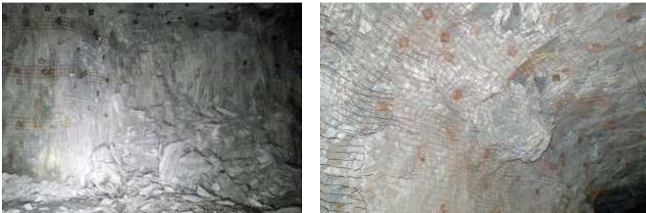
Figure 4. Strainburst a) ground support failed; b) the support retained the ground, Simser (2023).
