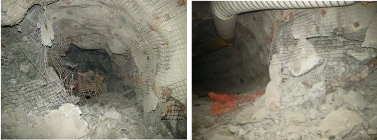
Figure 6. Damage following the January 2009 M_N 3.8, Counter (2014).
