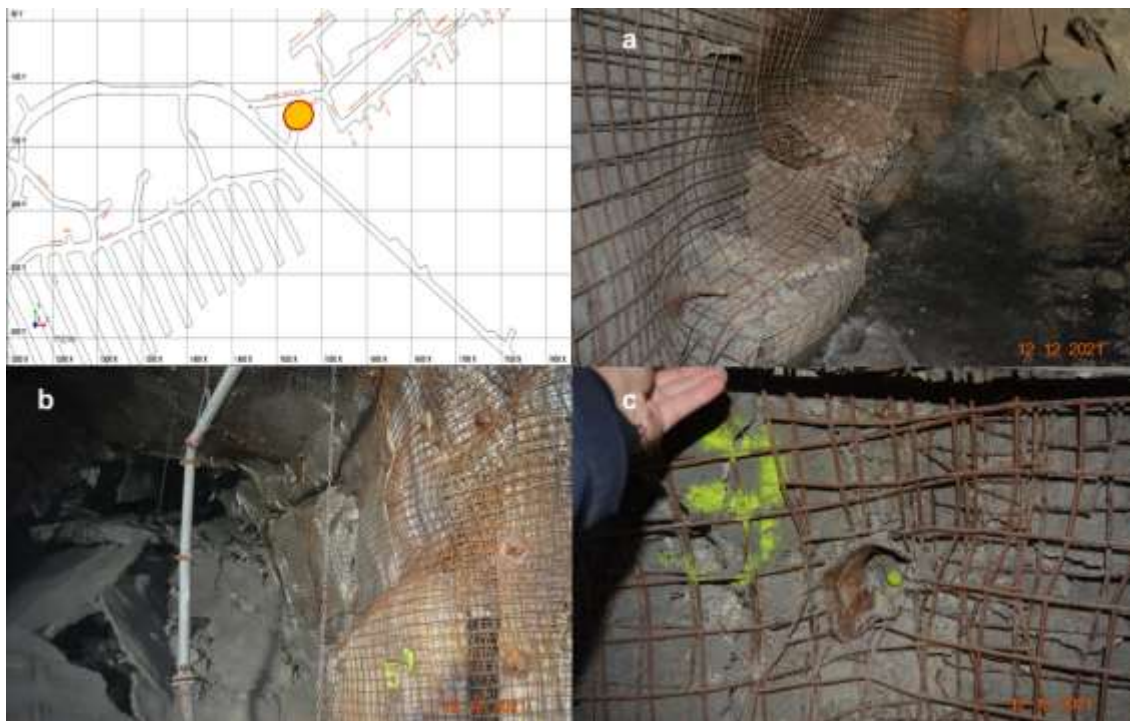
Figure 2. Example of damage observations in the LKAB Malmberget mine.
