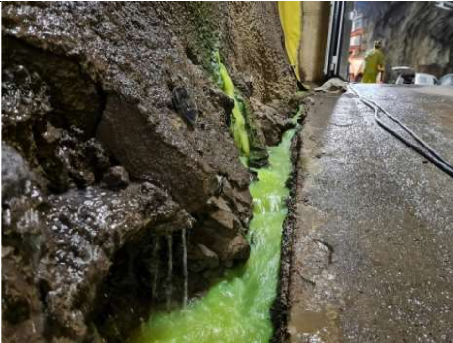
Figure 6. Clear connection between probe hole and leakage in the access tunnel during permeability test.
