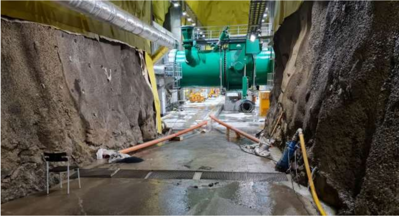
Figure 8. Provisional drainage system constructed on surface with open channel towards drainage tunnel to protect the permanent drainage system in the cavern.
