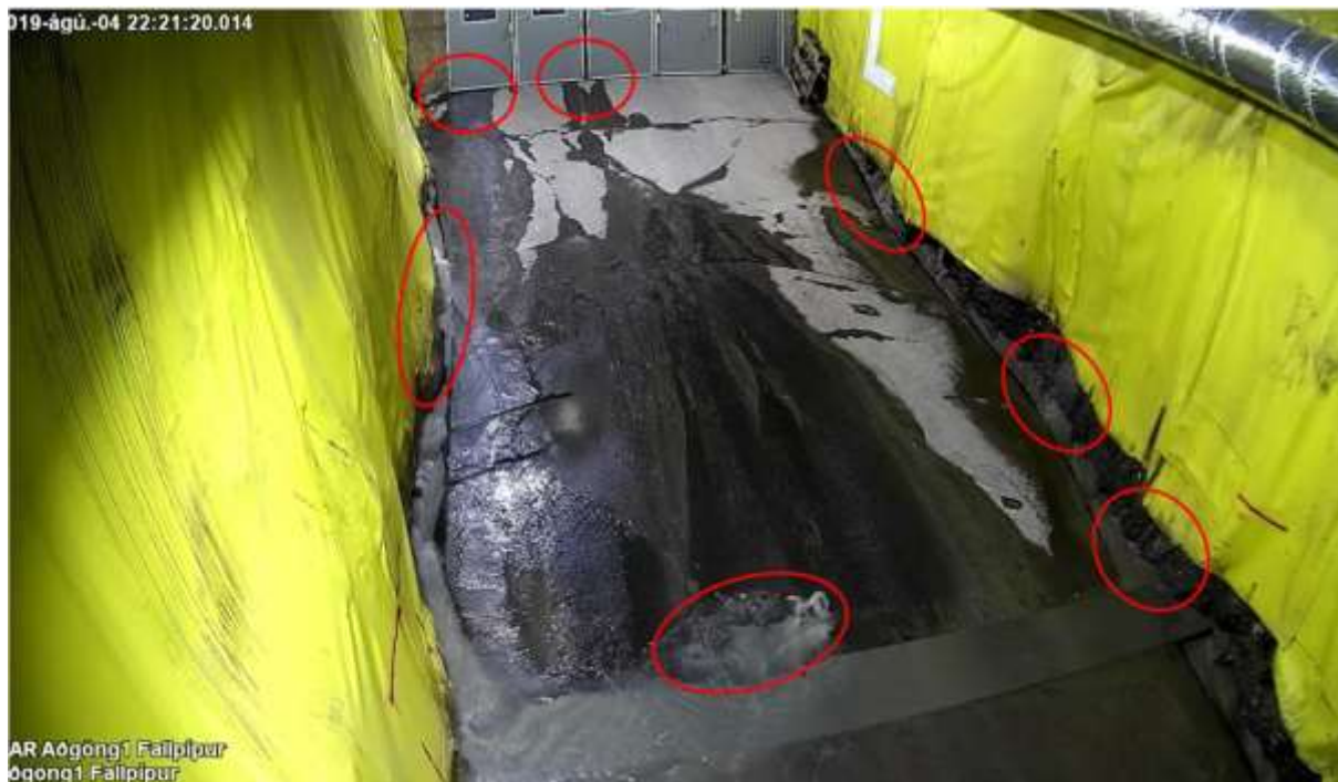
Figure 4. Observed increased leakage in access tunnel during a unit trip in august 2019. Note water flowing under portal door.
