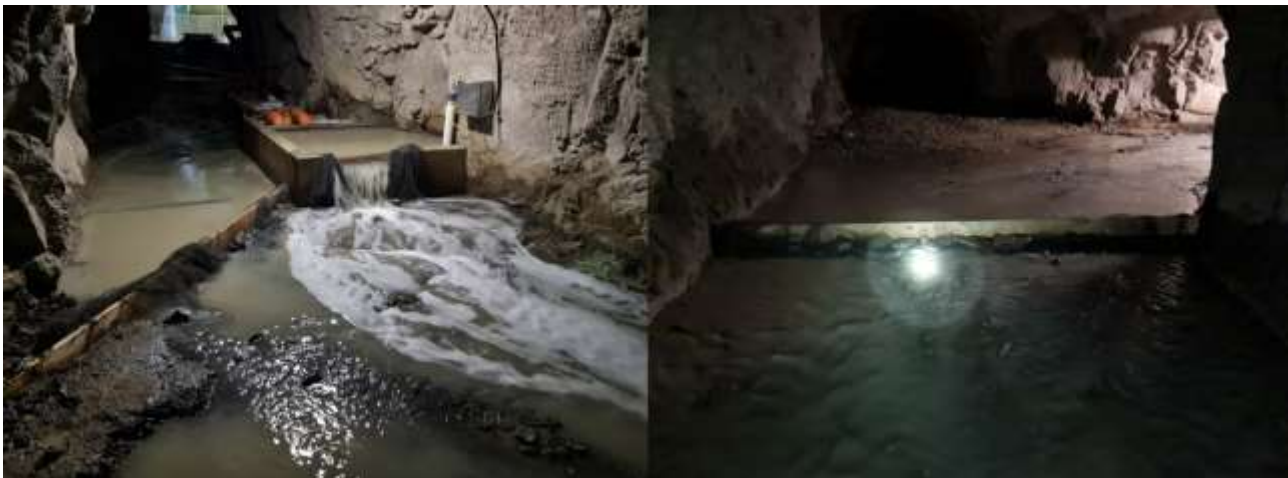
Figure 9. Measuring weir (left) and drainage tunnel invert installed with fishing net and wooden planks to catch reacted PU downstream the valve chamber.
