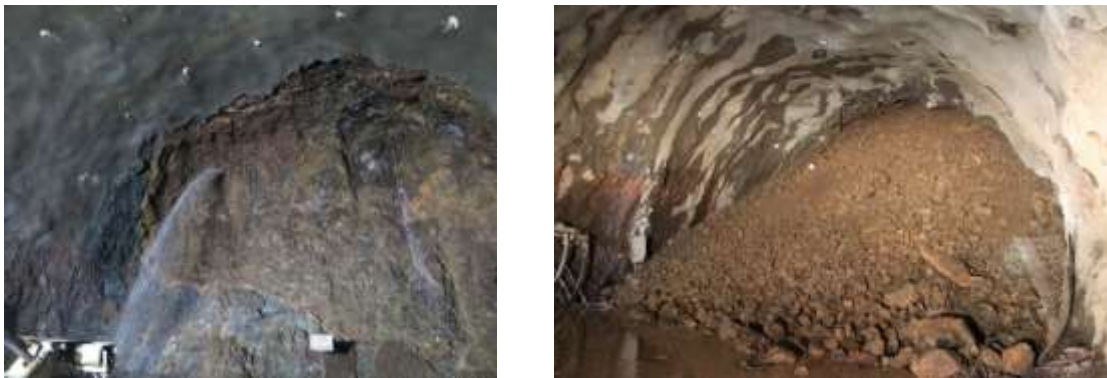
Figure 3. Collapse in the tunnel
