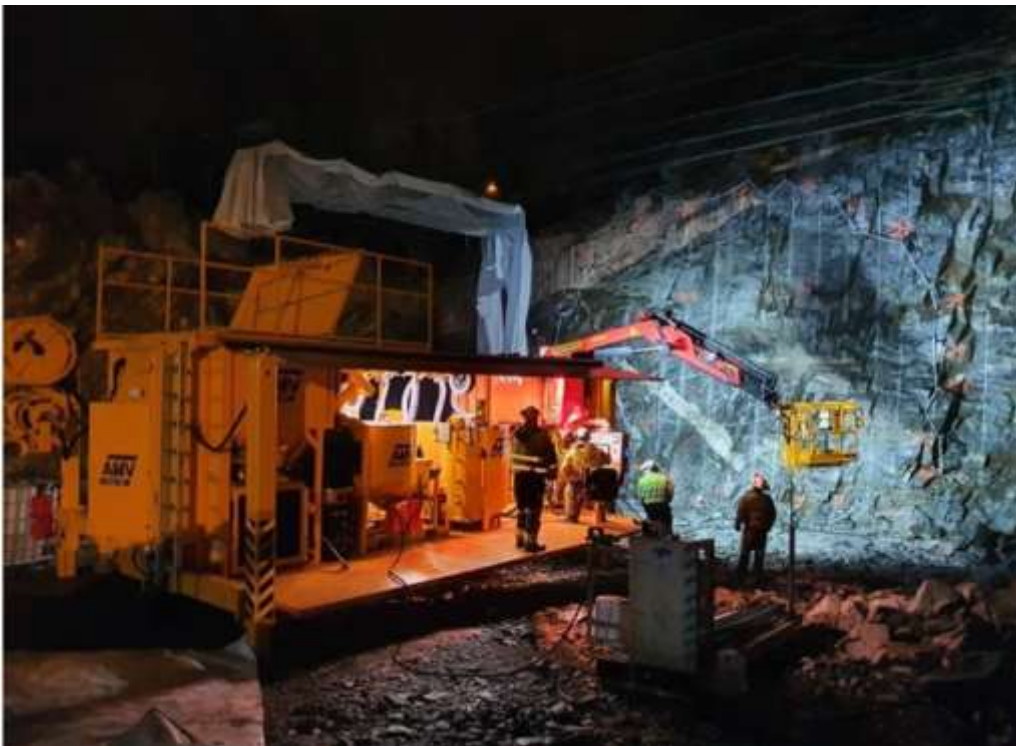
Picture shows preparations for pre-excitation grouting at Implenia/Acciona tunnel face in Moss. Picture by AMV
