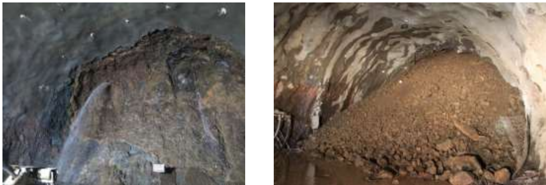
Figure 3. Collapse in the tunnel
